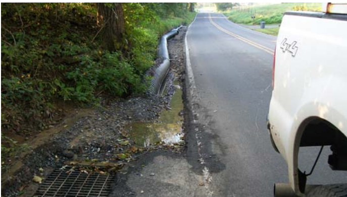
Blowout of Pipes along N. Fairville Avenue
